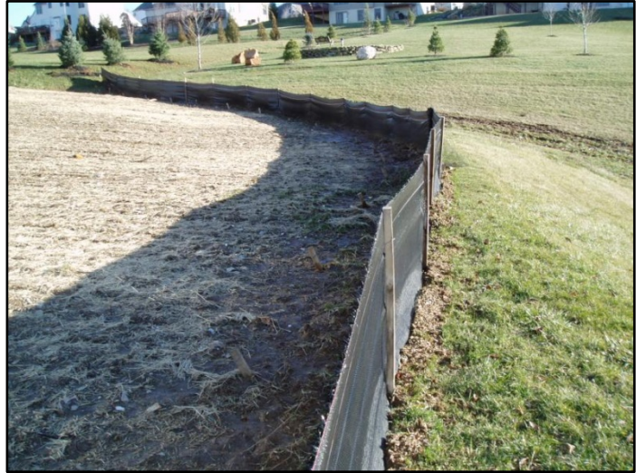
Figure 157. Silt fence (York County Conservation District 2009).
