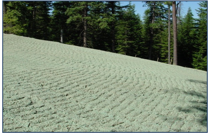
Figure 137. Exposed soil temporarily stabilized by roughening the surface ( North Idaho Hydroseeding ).
