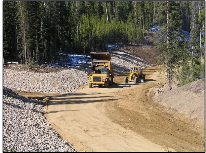
Figure 83. Placing new topsoil on Pioneer Mountain scenic byway, Orofino, Idaho ( Debco Construction ).
